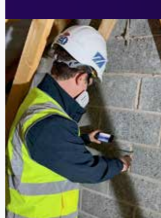
Health, Wellbeing & Safety Award Passive Fire Safety Measures
